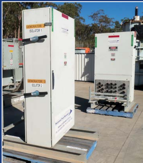
415V 800A & 415V 1600A switchboards
