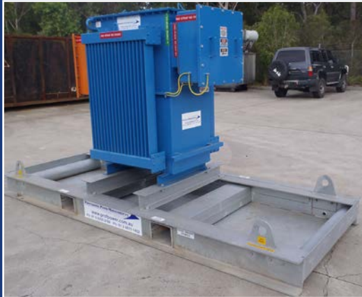
300kVA 1000 / 433V transformer on containment base
