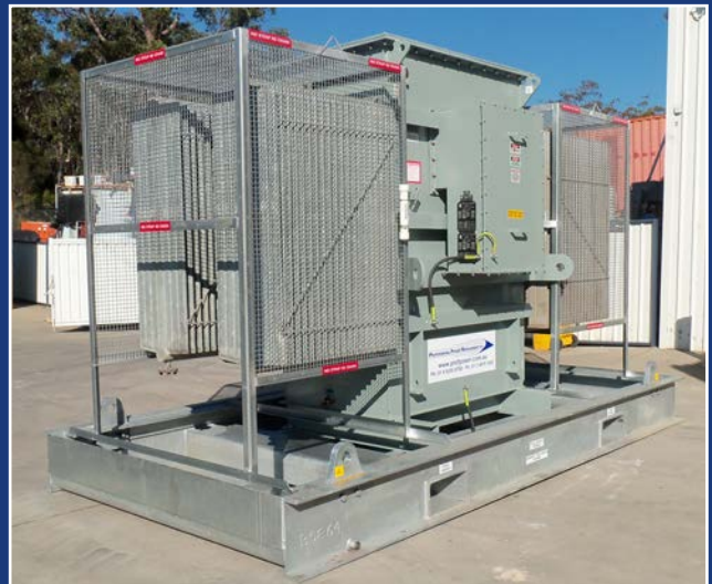
3325kVA 11000 / 6600V / 433V transformer on containment base
