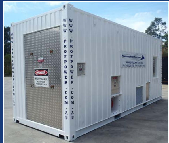
1600/2240kVA AN/AF 11000 / 433V substation with remote operable switchgear
