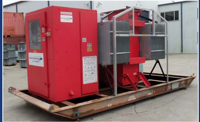
1500kVA 11000 / 435V substation with 11kV NER on containment base
