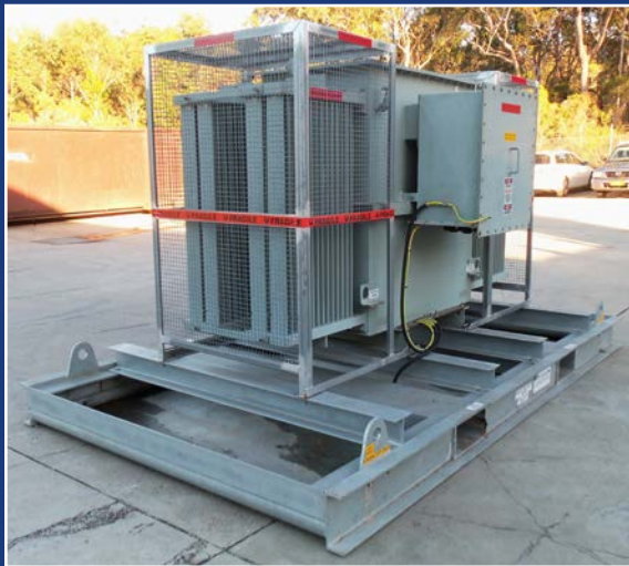
1500kVA 3300 / 433V transformer on containment base
